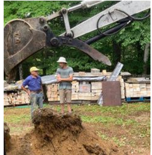
Al and Eric - foundation excavation and yet another brick moving day, July 2, 2022
